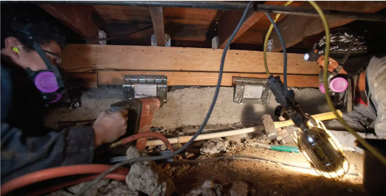
Noe Balderan, left, and Walter Gallaread of Bay Area Retrofit working to support an Oakland house's foundation. Credit...Peter DaSilva for The Bay Citizen
